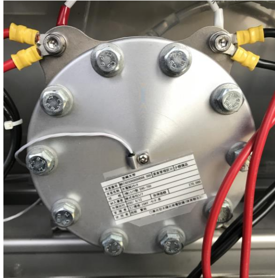
Fig. 2.7 Photograph of a PEM electrolyzer manufactured by Enoah Inc., EHC 070, installed at the University of Miyazaki.
