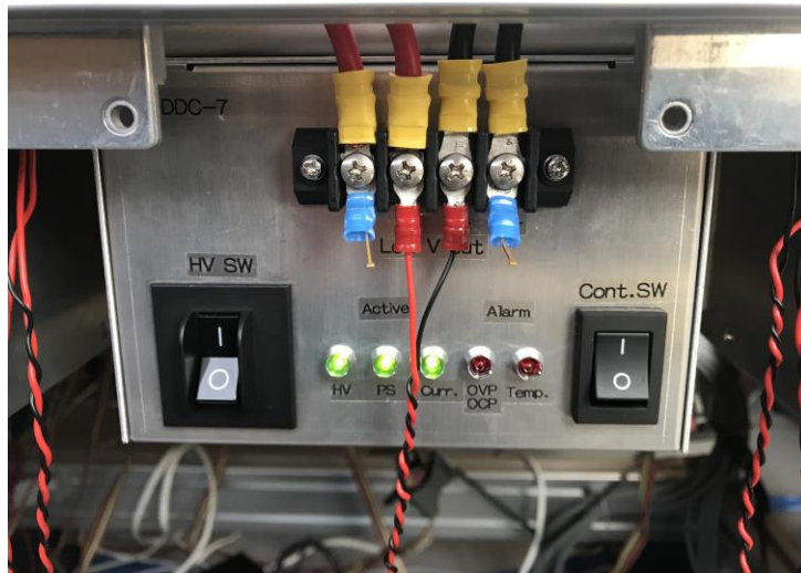
Fig. 2.5 Photograph of a DC/DC converter applied for the solar-to-hydrogen conversion.
