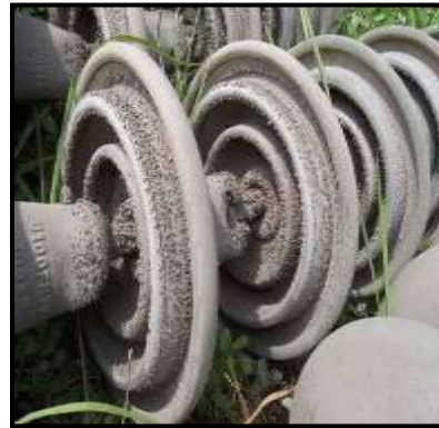
Figure 2. Insulator with cement vapor.
