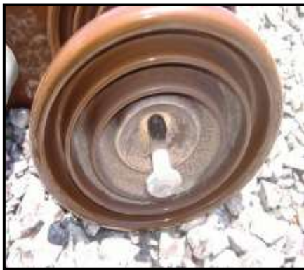
Figure 1. Removed Insulator with rust and corrosion.
