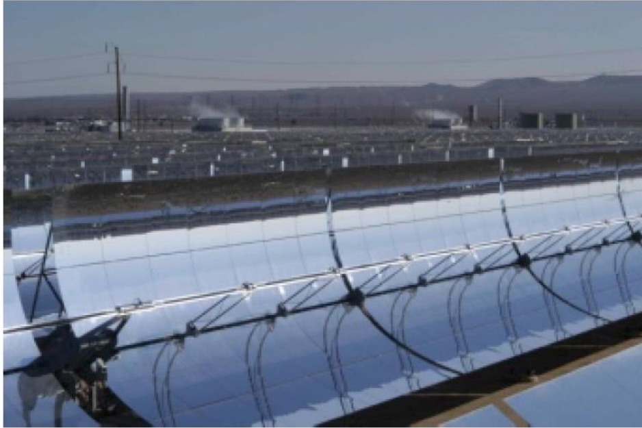
Fig. 1- 2: Photograph of the Eurotrough collector loop (Skal-ET) implemented by solar millennium California [2].
